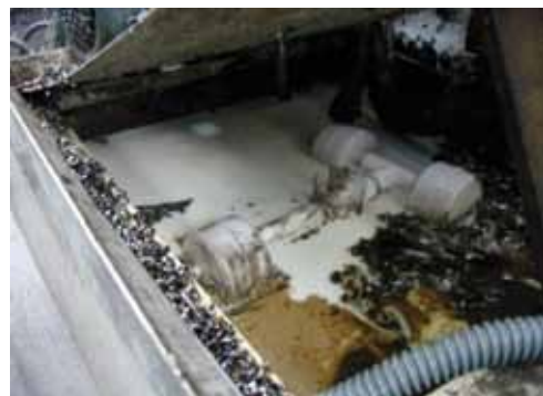
Vasca emulsione fortemente inquinata Coolant sump heavily contaminated
